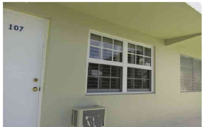
UNABLE TO IDENTIFY SEVERAL WINDOWS AS RATED
