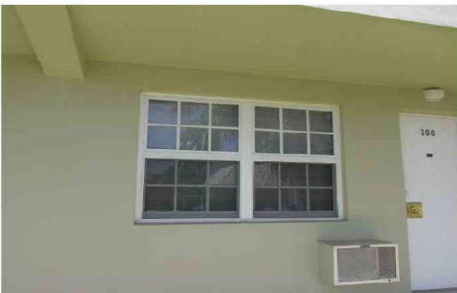
UNABLE TO IDENTIFY SEVERAL WINDOWS AS RATED
