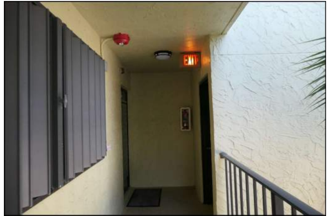
Photo 92 Fire Protection Systems
