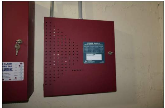
Photo 82 Fire Protection Systems
