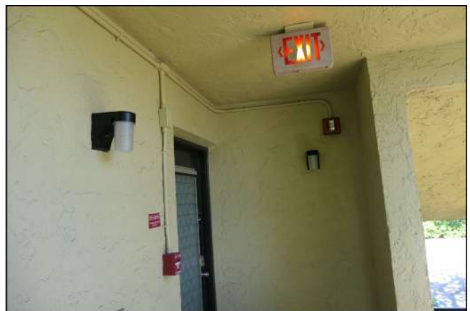
Photo 96 Fire Protection Systems
