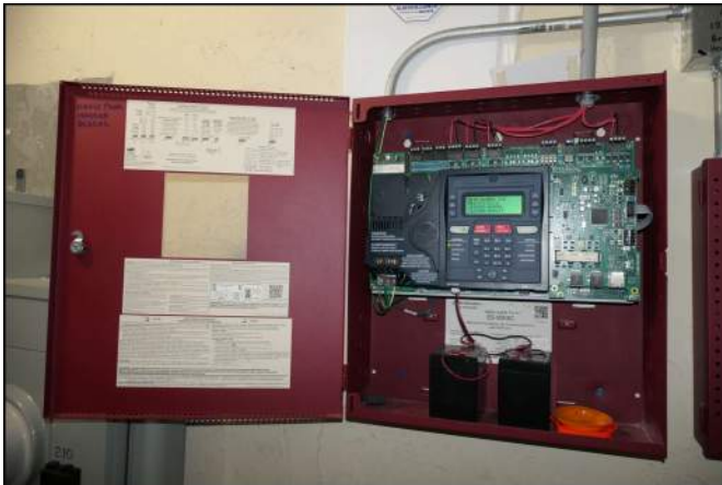
Photo 81 Fire Protection Systems
