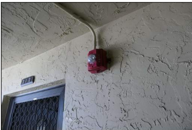
Photo 95 Fire Protection Systems
