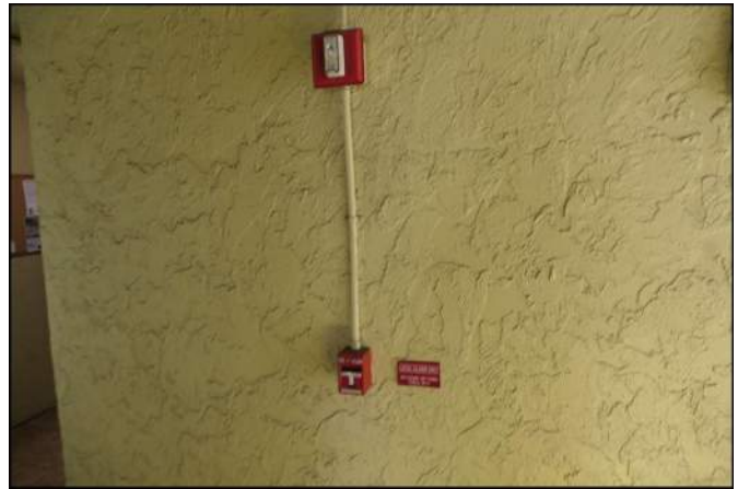
Photo 94 Fire Protection Systems
