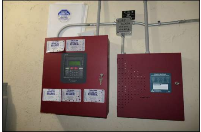
Photo 80 Fire Protection Systems
