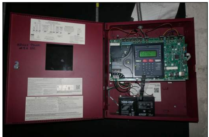
Photo 84 Fire Protection Systems
