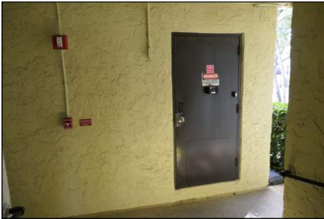
Photo 93 Fire Protection Systems
