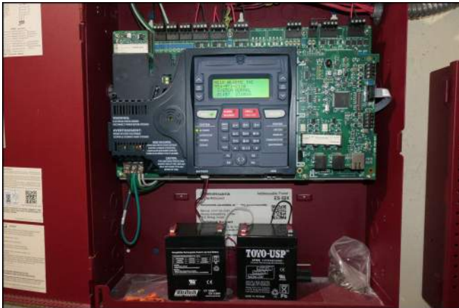
Photo 87 Fire Protection Systems
