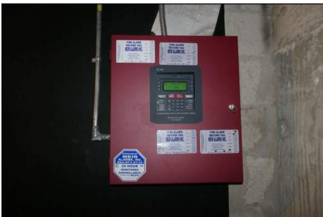
Photo 83 Fire Protection Systems
