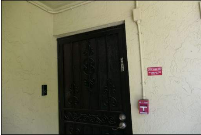
Photo 79 Fire Protection Systems
