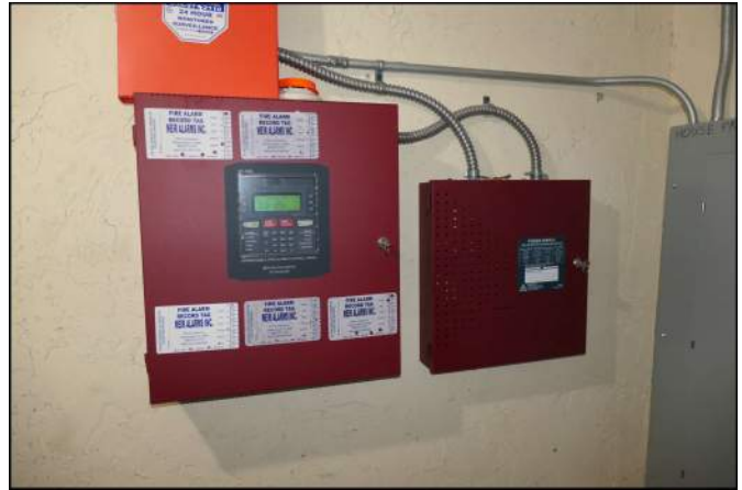
Photo 86 Fire Protection Systems
