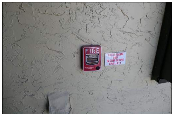
Photo 90 Fire Protection Systems
