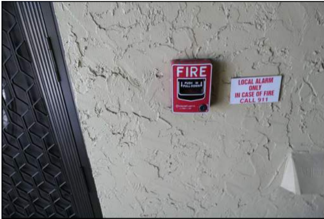
Photo 91 Fire Protection Systems
