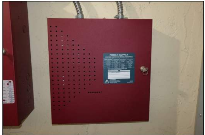
Photo 88 Fire Protection Systems
